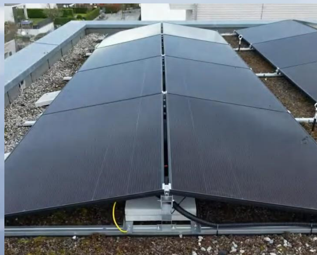
Ballasted mounting in Germany
