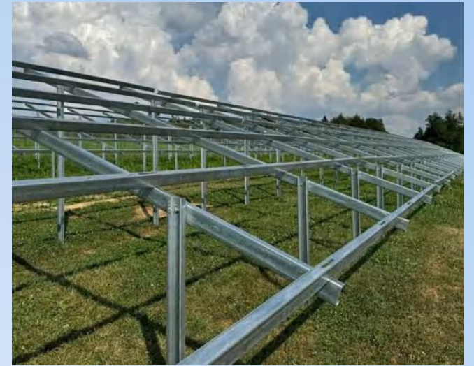
Steel ground mounting in Bulgaria
