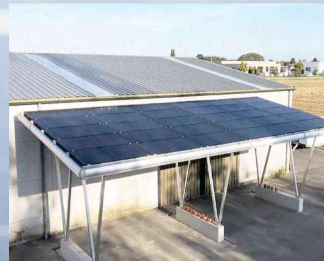
Aluminum solar carport in Italy
