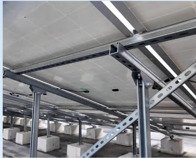
Ballasted mounting in China
