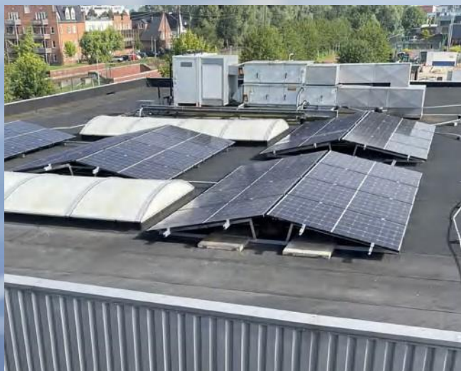
Ballasted mounting in Netherlands
